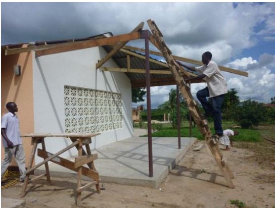
The roof of the car port had to be temporarily taken off.
