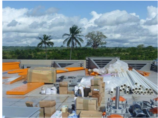
...of the material onto the flat roof of the school building.
