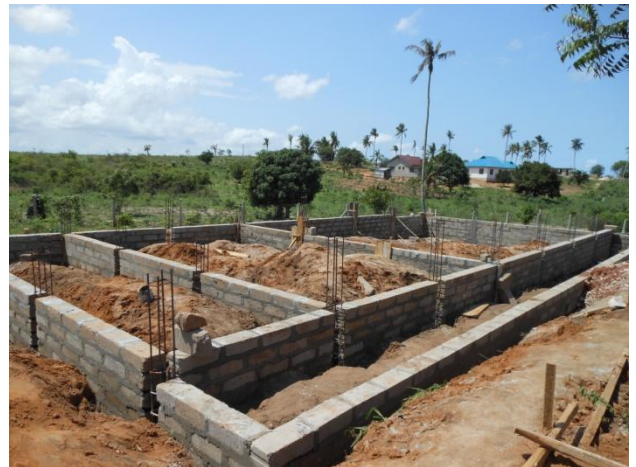
The construction of additional class rooms and the dining hall has started in November 2011.
